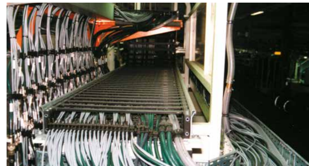
chainflex® CF5 and CF6 control cables (green) as well as CF211 measuring system cables (grey) in a screwing station of a motor factory. e-chain®: System E4/00 with chainfix clip strain relief devices
